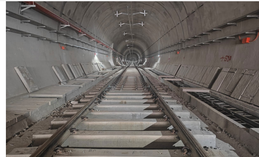
Tunnel Ventilation project, West Bengal
